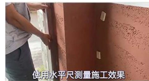
4.使用水平尺测量施工效果 Measure the construction size with a ruler
